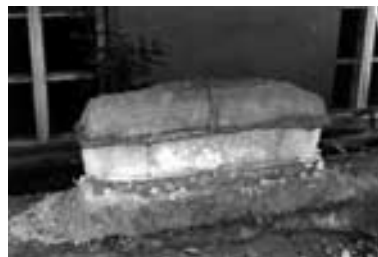
Not protected wall after three years of exposure to external weather conditions
